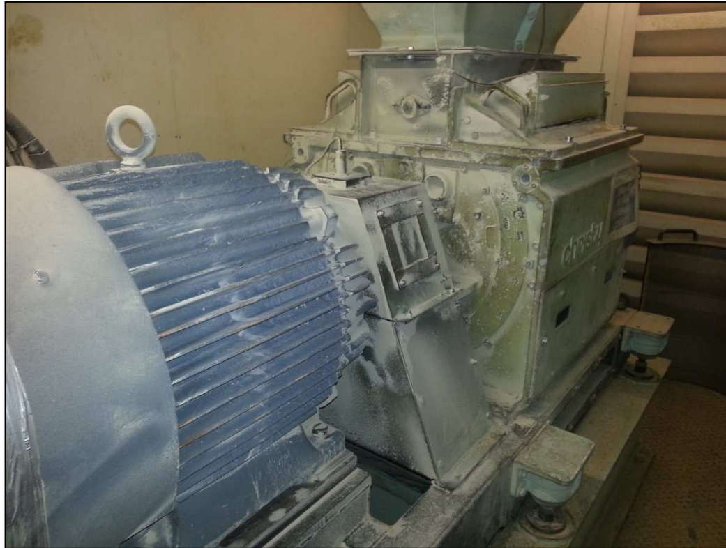
Hammer Mill – Motor Bearing Damage
